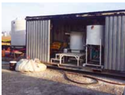
Surface grout plant. Due to the space constraints and logistical issues associated with the underground space, all cementitious grout was mixed on the surface and pumped via slicklines for underground injection.
