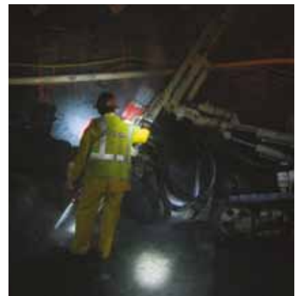
Grout hole drilling performed using an Airtrack drill rig. Drill through packers were used so that large volumes of water could be controlled if encountered.
