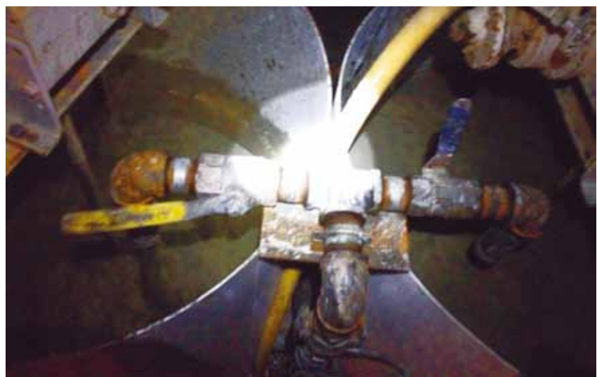
Microfine grout being delivered to the underground agitation/pumping plant.
