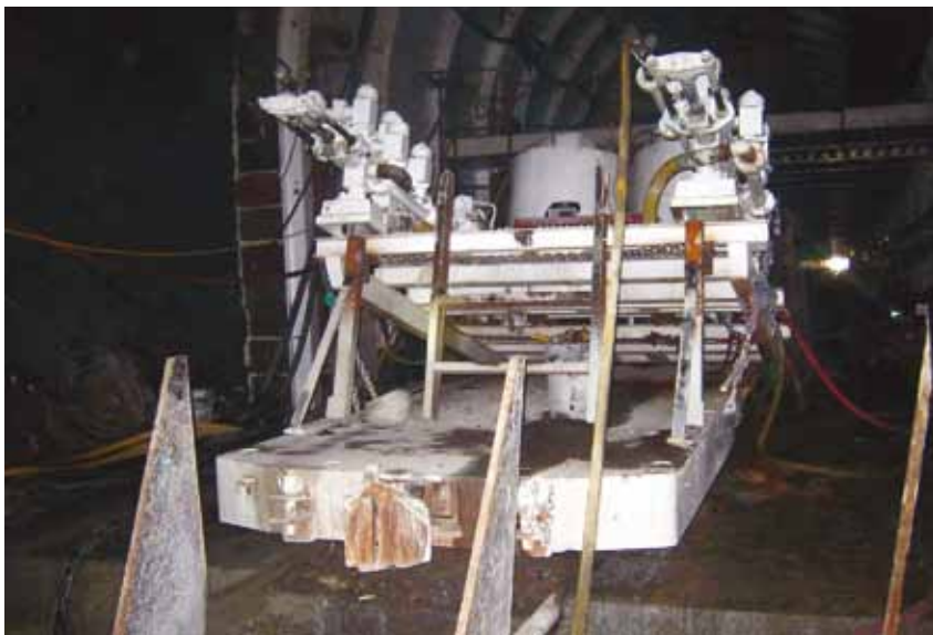
Underground agitation/pumping plant. All cementitious grout was mixed on the surface and delivered underground for injection. Once underground, the grout was continuously agitated and pumping rates and pressures could be more precisely controlled than if grouting was conducted via surface pumps.
