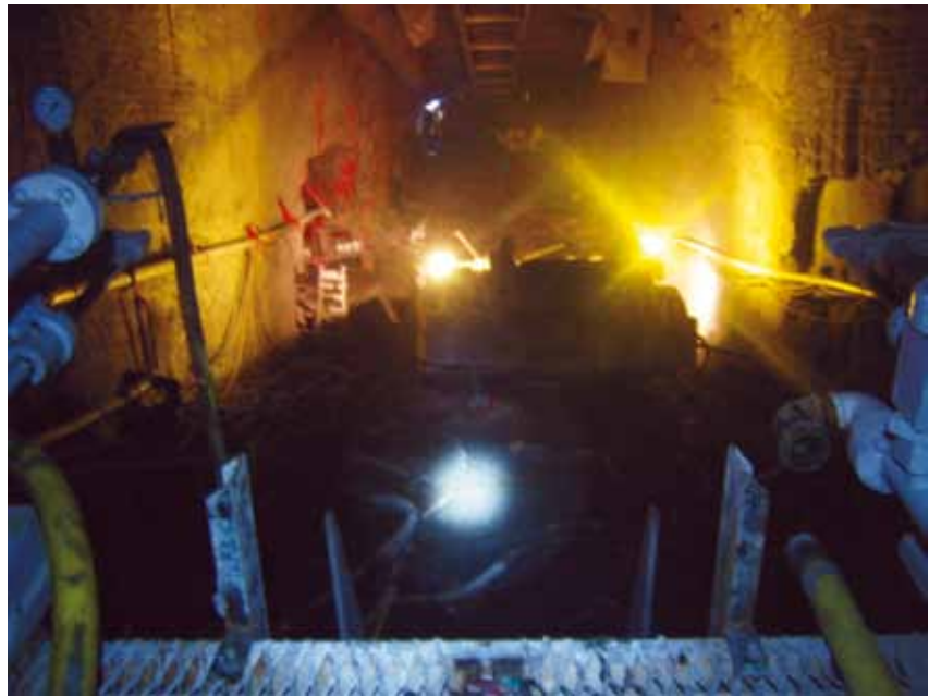
View from the platform of the agitation/pumping plant looking toward the working face. The underground pumping operation was generally 200 – 300 ft from the injection point. This was because the plant could easily be moved on rail to the end of the finished invert and because the area between the end of the finished invert and face was highly congested with mining equipment and grout hole drilling equipment.
