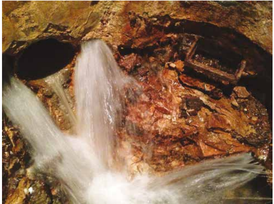
Groundwater infiltration through cracks in a manhole.
