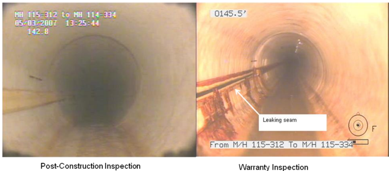
Figure 6. Seam Leakage evident over time
