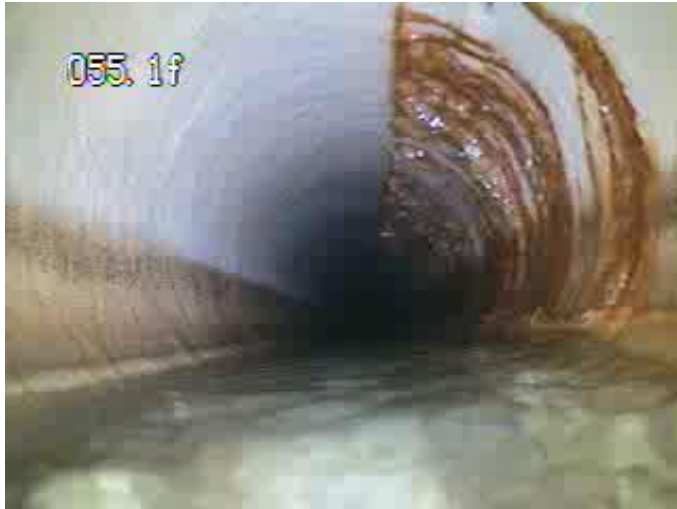
Figure 5. Seam Leakage on lateral liner
