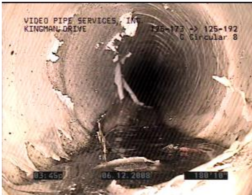
Figure 7. Lateral liner coating delamination
