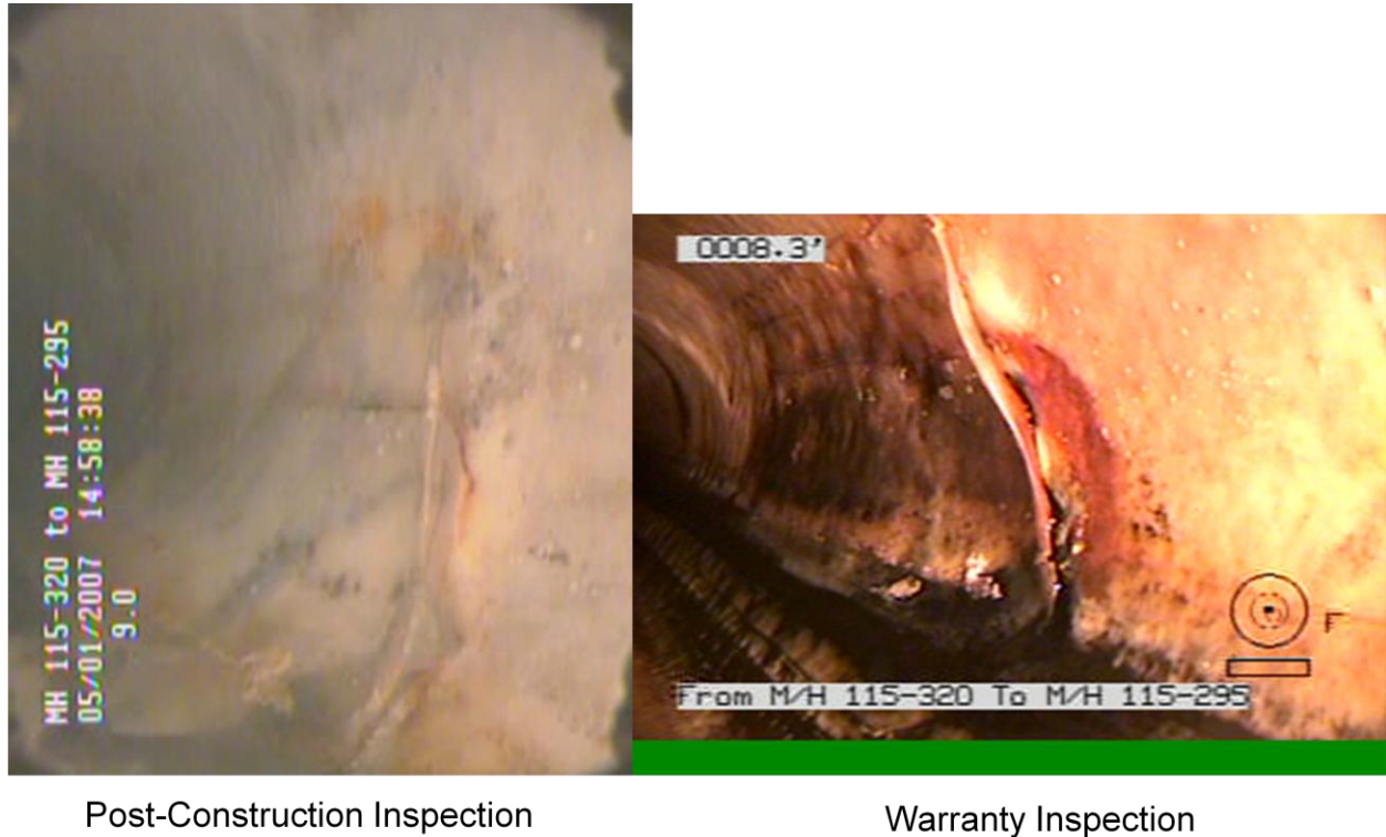
Figure 10. Detached Factory Patch Found at Warranty Inspection
