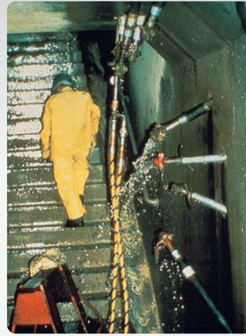
Leaking gallery stairs prior to repairs. Notice the high presence of water.
