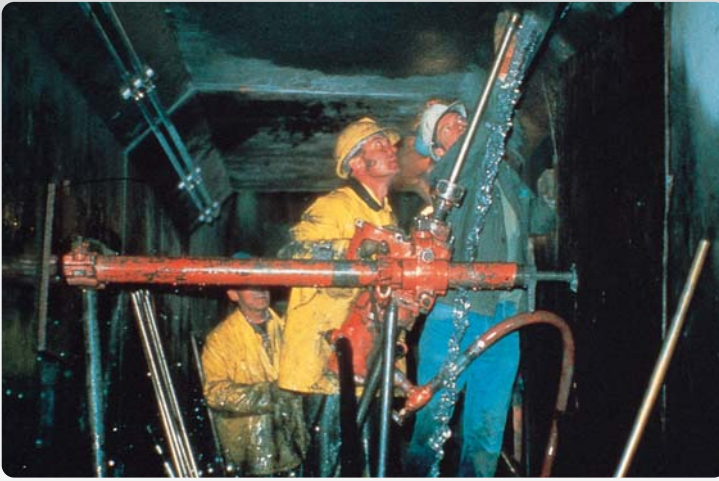
Interior of dam tunnel. Drilling into joint intersection with leg drill; water swivel using extension pipe for depth.
