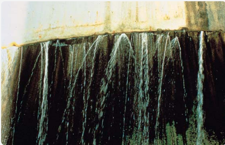
Water leaking through dam.
